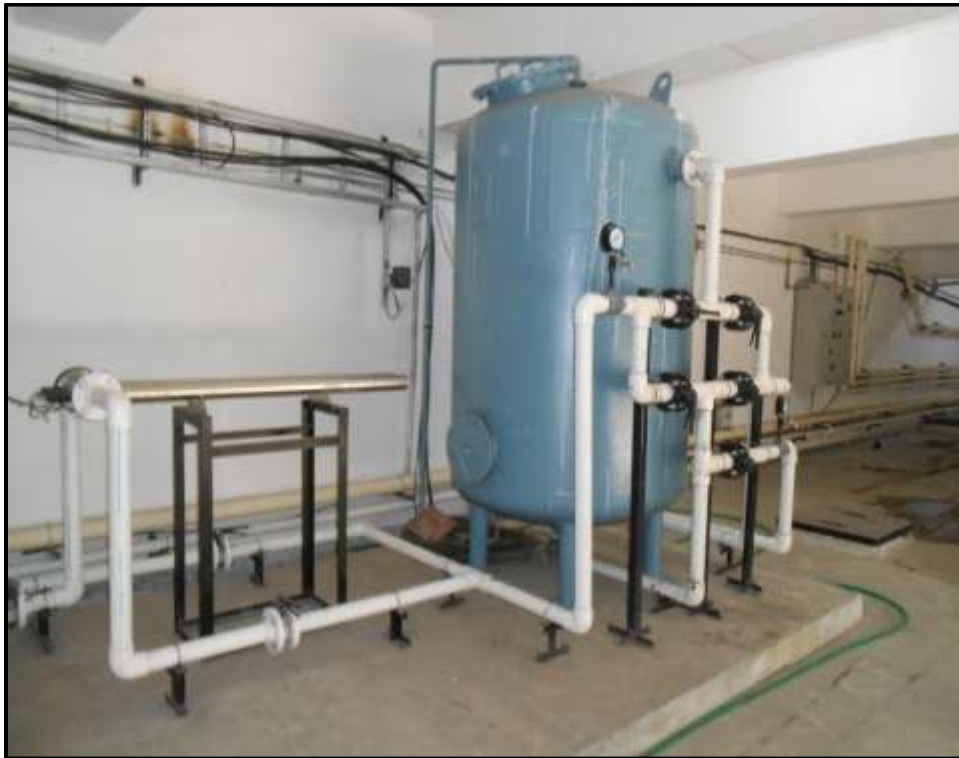
Activated Carbon Filter & UV Filter
